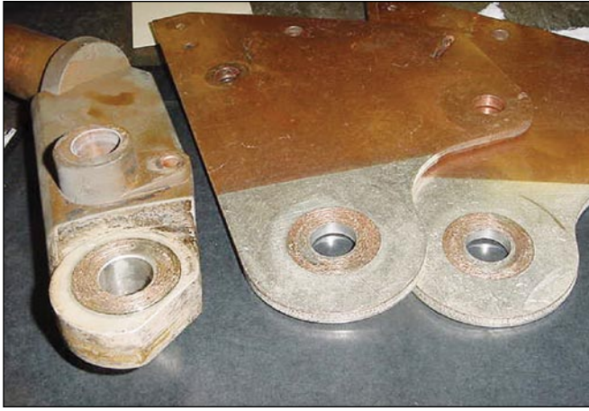
Figure 3 — Siemens MA-250 Contact Pivot Point Wear
